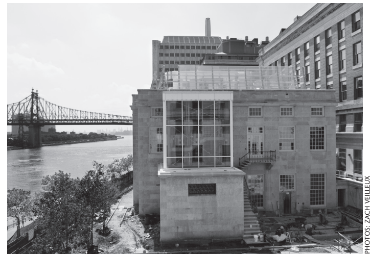
Move-in condition. Construction is nearing completion on the first floor of Flexner (top) and the exterior of Welch. For more photos, visit benchmarks.rockefeller.edu .
