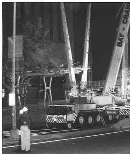
RU's new pedestrian bridge was put into place last Sun., Oct. 3. Photo by Joseph Bonner
