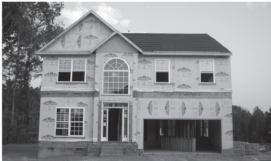
Headed south. Michael John's new home, in Wake Forest, North Carolina, during its construction. Mr. John's wife, Martha, has been living there since 2005.
