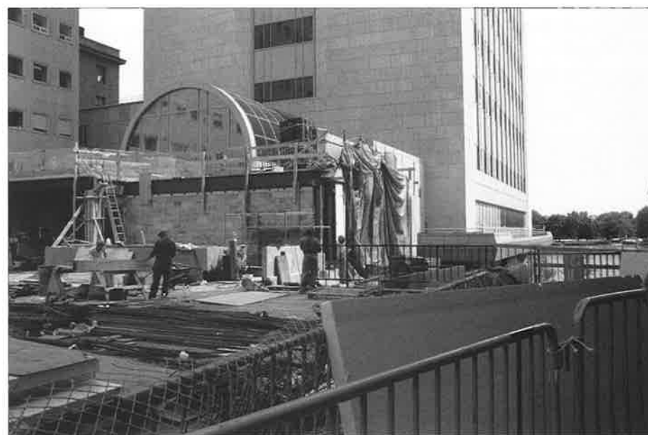
The plaza construction progressed over the summer, with the infrastructure for a raised plaza level, tree grove and fountain area with an accompanying grass slope to the entrance of Weiss taking shape. Photo by Pavani Thagirisa.
