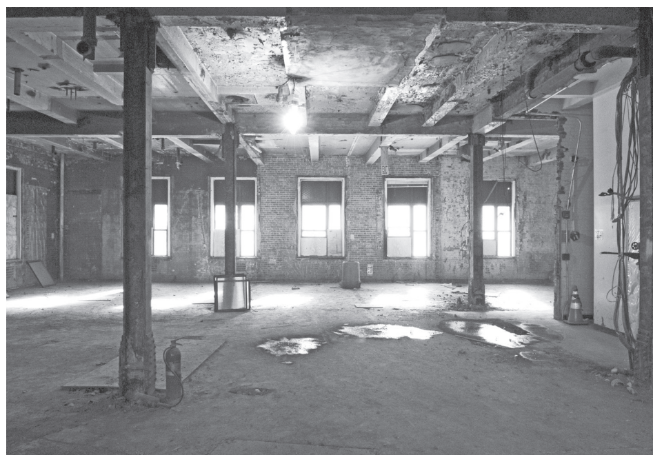
Demolition. The first floor of Flexner Hall, fully demolished and ready for the next phase of construction. This space, at the east end of the building, was formerly occupied by the Tomasz Lab.
